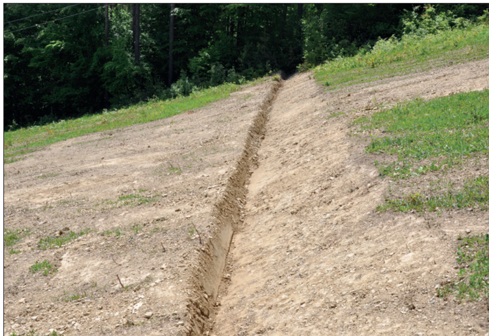
Fig. 9. Erosional incisions at the outlet of a drainage ditch from the ski run, Kotelnica Białczańska
