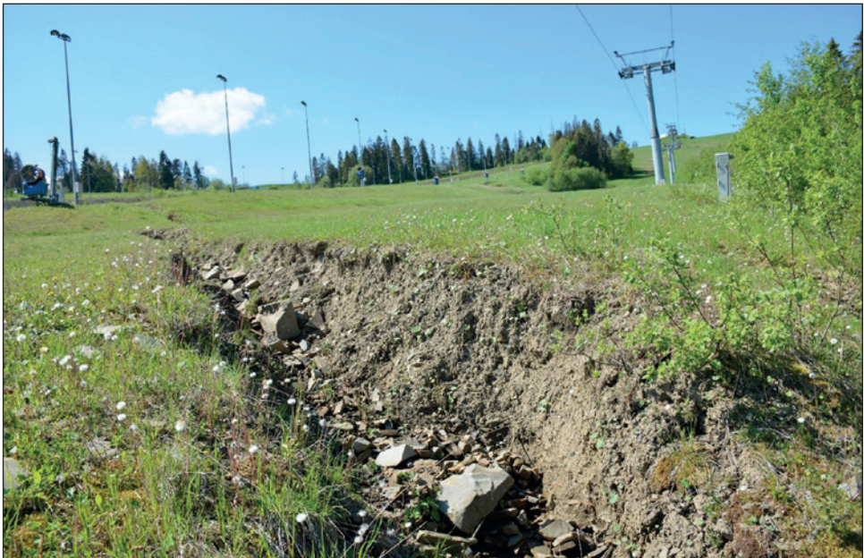
Fig. 8. Diagonally routed drainage ditch, Kotelnica Białczańska
