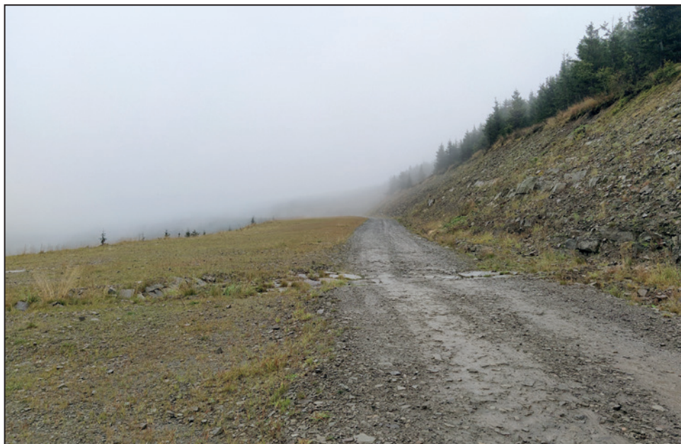
Fig. 13. Ski run in the Skrzyczne massif. Visible road undercut and escarpment, surface without vegetation and the road running in the ski run area. Drainage ditch is masonry with large stones
